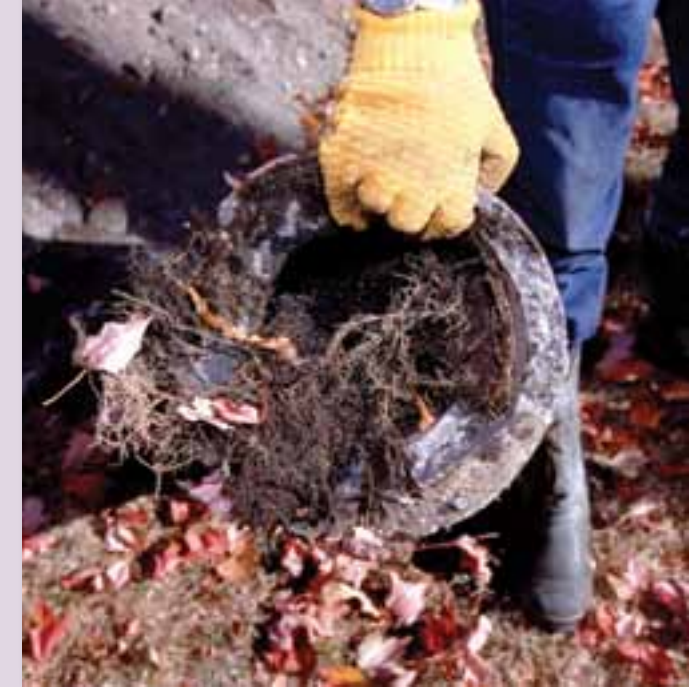
Roots from trees and bushes are a common cause of clogged side-sewer lines. Roots can easily penetrate pipes made of porous concrete such as this one, which is more than 25 years old. Modern side-sewer lines are made of heavy duty, water-tight plastic and therefore last much longer.
