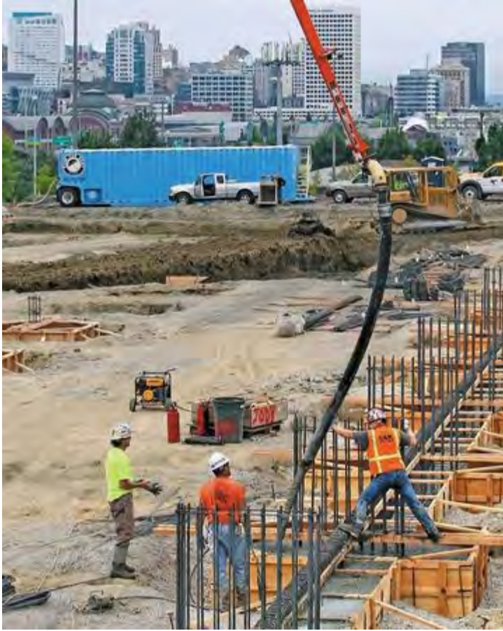
DEAN J. KOEPLER/STAFF PHOTOGRAPHER - JTM Construction workers pour part of the foundation of the LeMay museum Thursday. Sixty-five Cal Portland Concrete truckloads were used that day to pour the two mat footings and two-thirds of the building's foundation. The car museum will occupy 165,000 square feet of space in what once was the Dome's B and C parking lots.
