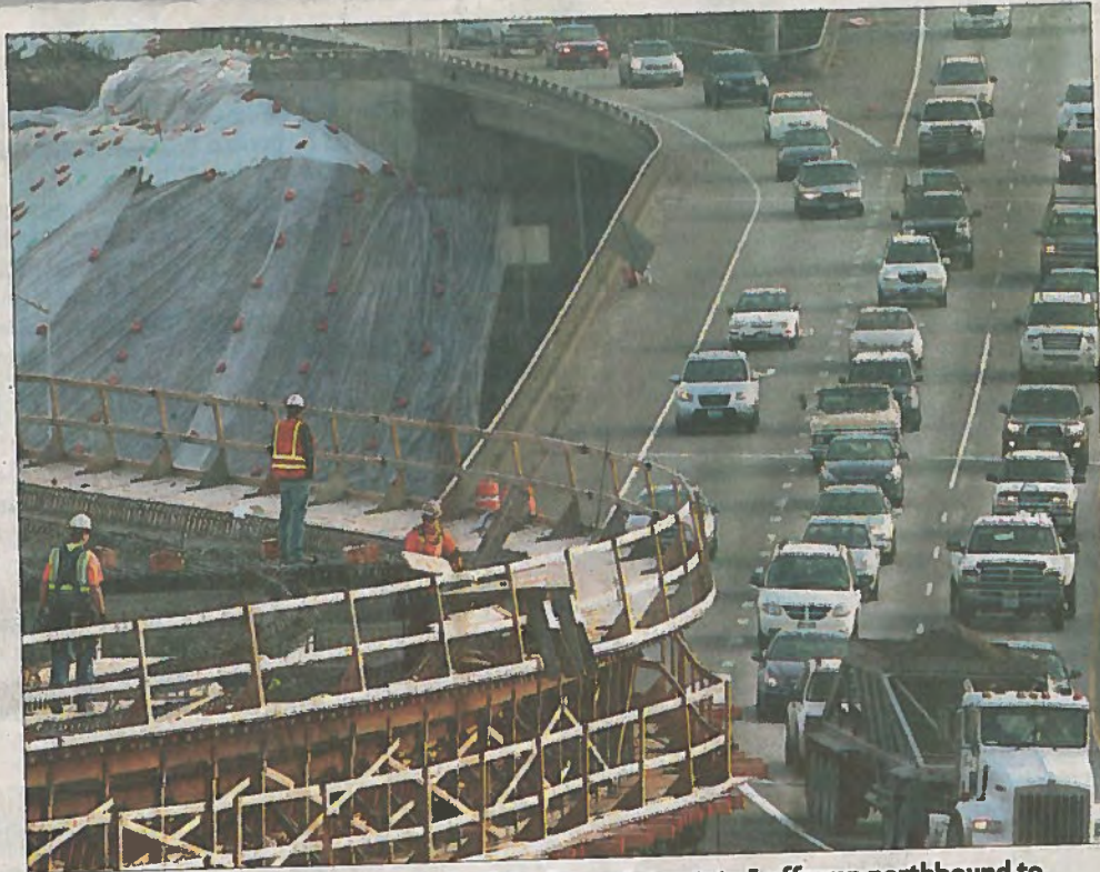
Workers build forms for roadway slab of the future Interstate 5 offramp northbound to Sprague Avenue. Their perch gives them a bird's-eye view of traffic on the existing Nalley Valley viaduct this week.
