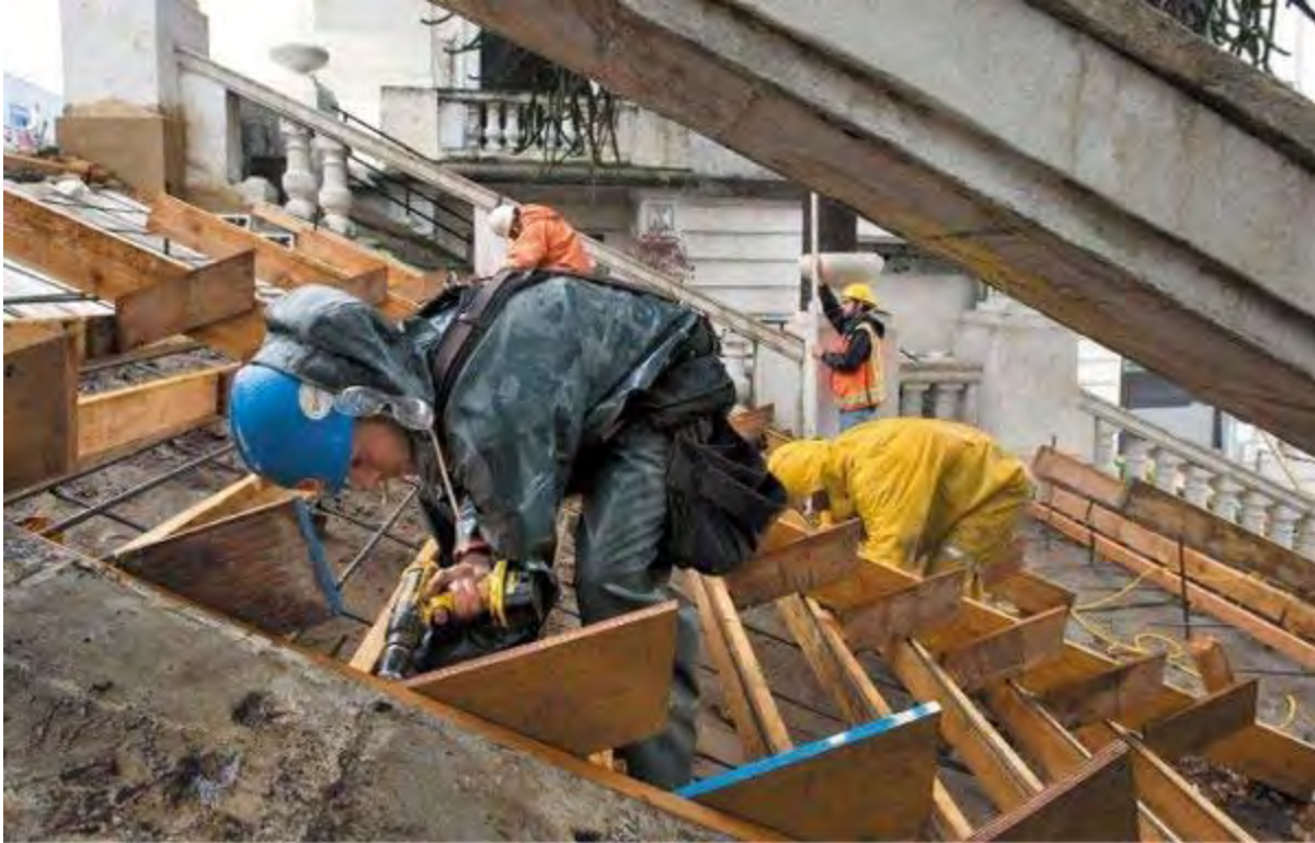
PETER HALEY/ STAFF PHOTOGRAPHER - Construction workers, including carpenter's apprentice Brian Pease of Edgewood, foreground, prepare forms for pouring concrete steps Friday, part of the rebuilding of the Spanish Steps adjacent to the old downtown Tacoma Elks building, which is being redeveloped by McMennamins. Order News Tribune reprints Order Associated Press reprints
