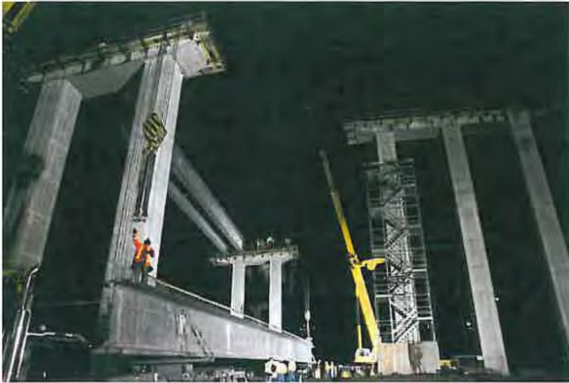
Staff photographer - After two girders are already in place atop columns, left, a worker reaches to strap a third girder to cranes that will lift it more than 70 feet a top the columns, in Tacoma, Wednesday night. By summer 2011, when the new highway 16 westbound viaduct lanes open, 220 girders will be used to form the roadway.
