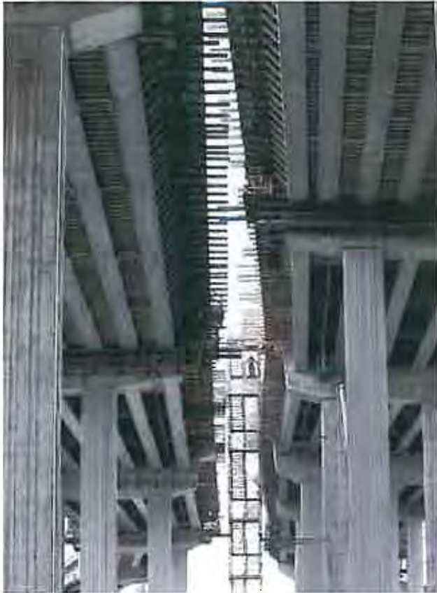
DEAN J. KOEPFLER/STAFF PHOTOGRAPHER - A worker climbs a construction tower last week to work on the new lanes of westbound state Route 16, left, and the new ramp from southbound Interstate 5, right, supported by massive piers on Center Street in Tacoma.
