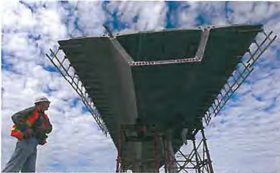
The Olympian - Les Dubois, an engineer with the state Department of Transportation, inspects a cantilevered section of a bridge Wednesday that will carry vehicles from northbound I-5 to westbound state Route 16 and to the Sprague Street exit.
