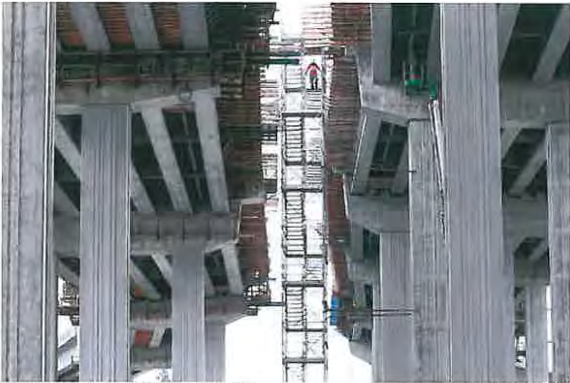
Staff photographer - A worker climbs a construction tower last week to work on the new lanes of westbound state Route 16, left, and the new ramp from southbound Interstate 5, right, supported by massive piers on Center Street in Tacoma.
