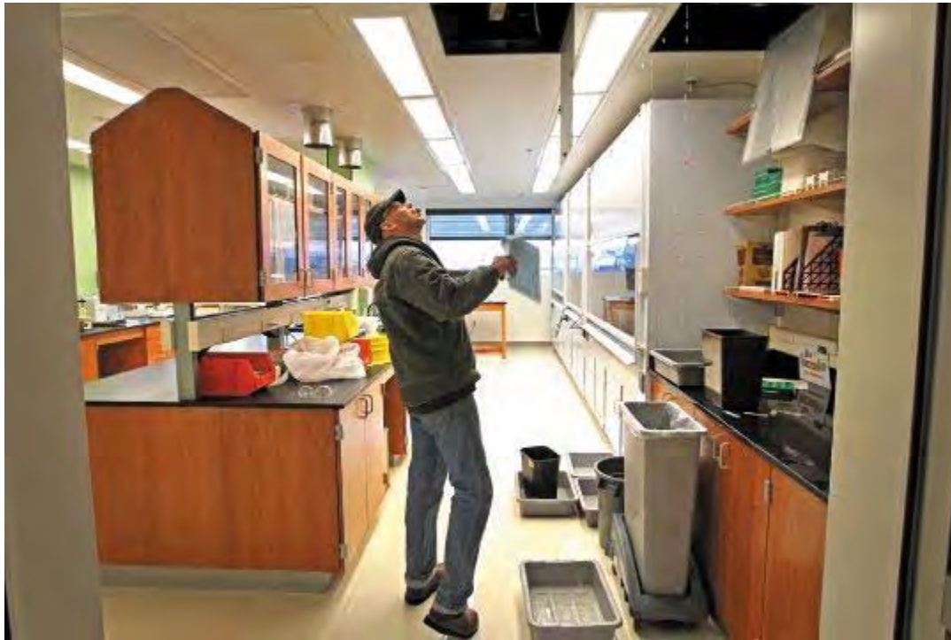
DEAN J. KOEPFLER/STAFF PHOTOGRAPHER - Geoffrey Smyth, manager of environmental services for the City of Tacoma, looks up into water leaking from the ceiling of a thirdfloor lab at the Center for Urban Waters building.
