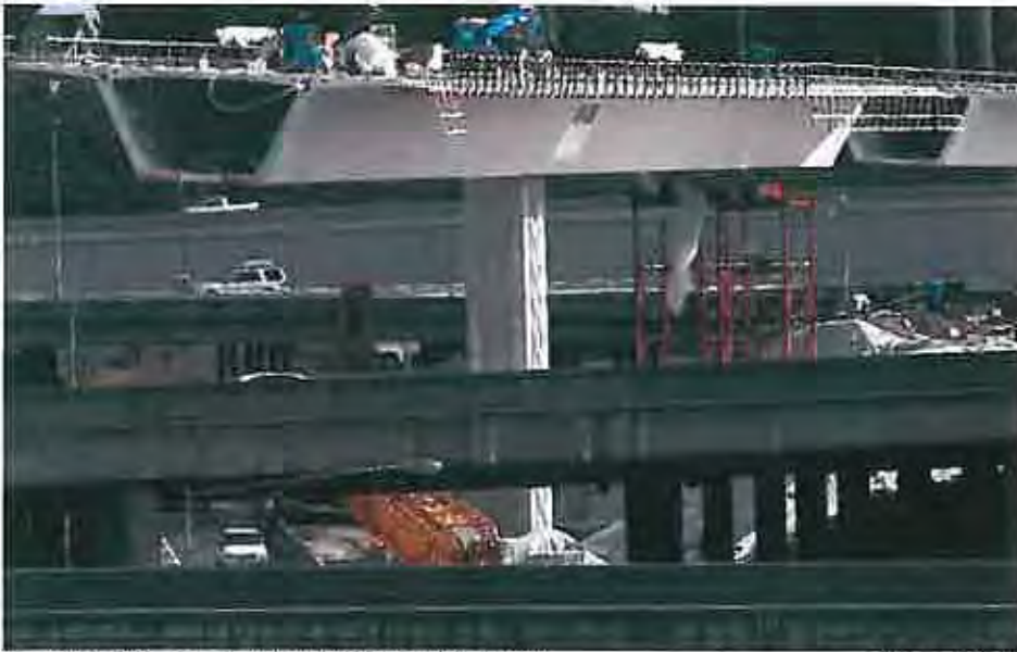
The Olympian - Cantilevered bridge sections tower over ramps and overpasses in Tacoma's Nalley Valley. Twenty-two concrete sections weighing as much as 80 tons are cantilevered of 100-foot-high supports. When finished, the bridge will carry traffic from northbound I-5 to westbound state Route 16.
