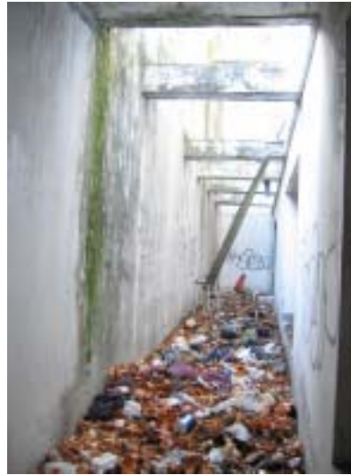
CP. 5.2.18 Debris filling areaway. Note exposed rebar in braces spanning between Spanish Steps (left) and Elks Building (right).
