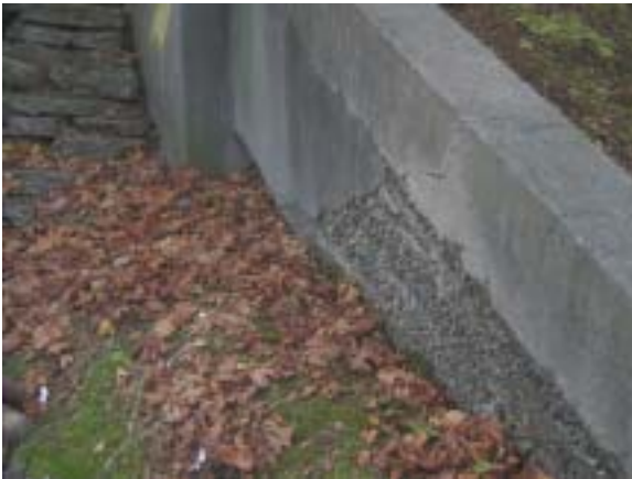
CP. 5.2.20 Southwest retaining wall. Exposed aggregate portion was formerly covered by grade. Height of exposure suggests extent of slope settlement.
