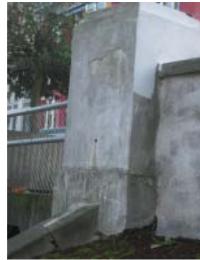
CP. 5.2.10 Delamination of previous parging added on the newels. Note weep hole drainage redepositing dissolved cast stone along top of retaining wall.
