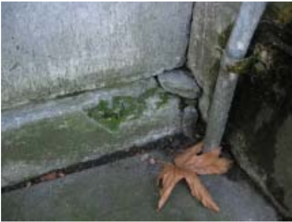
CP. 5.2.14 Cracking along newel base.
