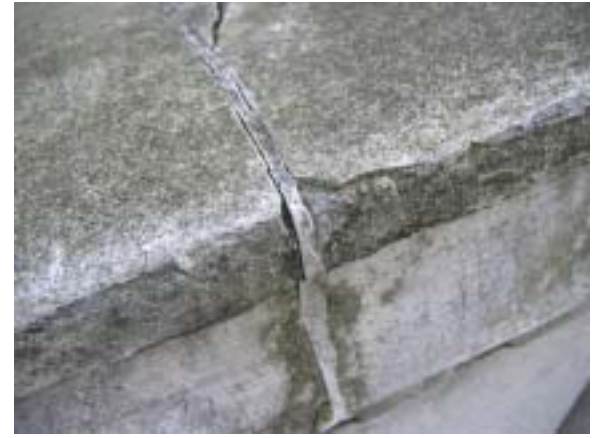
CP. 5.2.7 Separation of previous non-compatible caulking from railing.
