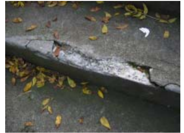
CP. 5.2.16 Deteriorated and previously repaired stair nosing.
