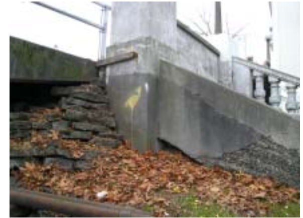
Photo No. 2: Detail of grade settlement at south slope (southwest corner). Source: PCSA Structural Solutions.
