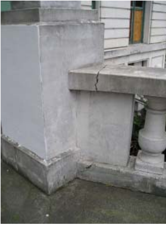
Photo No. 1: Detail of arced railing and newel joint. Note crack at connection. Source: PCSA Structural Solutions.
