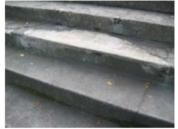
CP. 5.2.13 Previous cementitious stair repairs.
