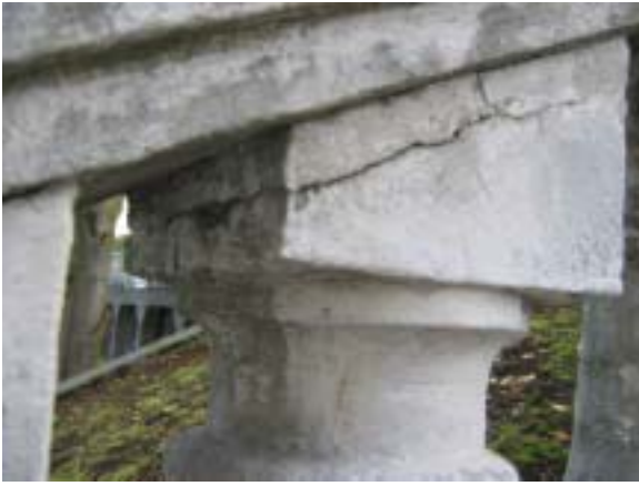
CP. 5.2.5 Cracking along the upper portion of a baluster.
