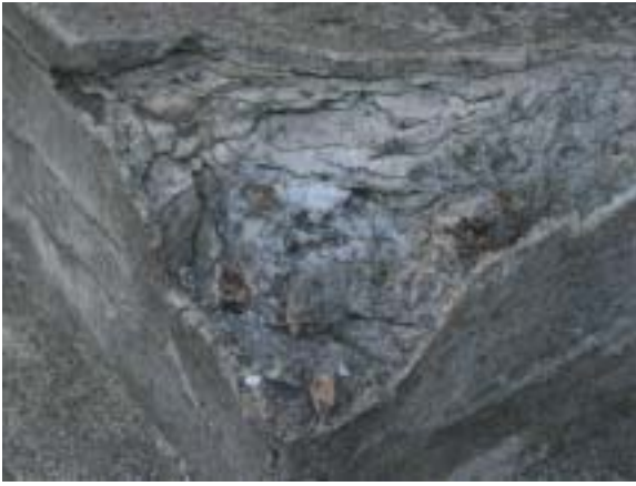
CP. 5.2.11 Deteriorated upper corner on a typical newel.
