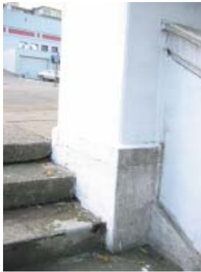
CP. 5.2.9 Lateral crack along base of upper northwest newel.
