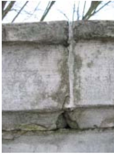
CP. 5.2.6 Cracking and previous non-compatible caulking employed at joints in railings.
