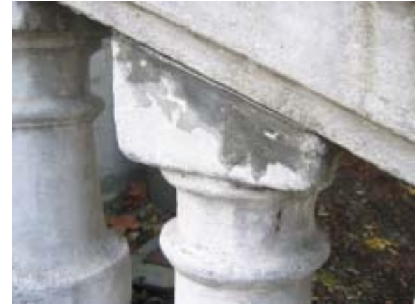
CP. 5.2.2 Previous, non-compatible contemporary patches to the balusters.
