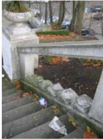
CP. 5.2.1 Missing balusters along the south portion of the upper stairs. Note grade of planting area behind balustrade approximately at stair level.
