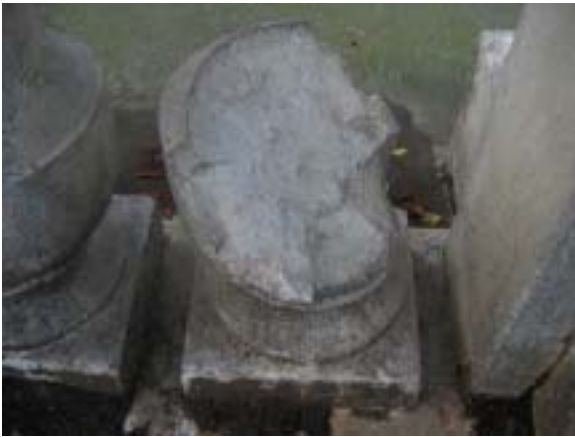
CP. 5.2.8 Broken cast-stone baluster.
