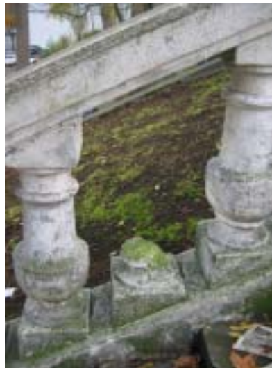
CP. 5.2.3 Missing baluster along the south portion of the upper stairs. Note grade of planting area behind balustrade approximately at stair level.
