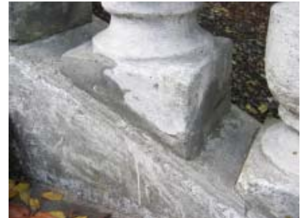
CP. 5.2.4 Previous, non-compatible cementitious patches to the balusters.
