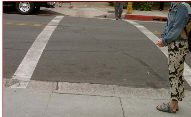
Parallel markings are the most basic crosswalk marking type, and are applied where textured concrete crosswalks are used
