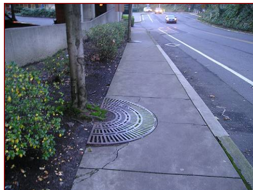
Tree well grates can create uneven sidewalk conditions
