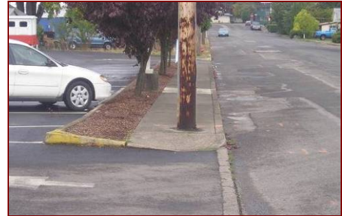
Narrow sidewalks can often be blocked by utilities
