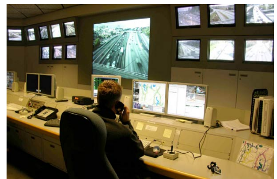
WSDOT Seattle Area Traffic Management Center
