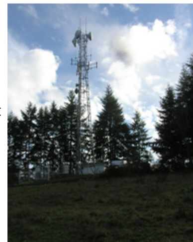
WSDOT Wireless 800 MHz Radio Tower
