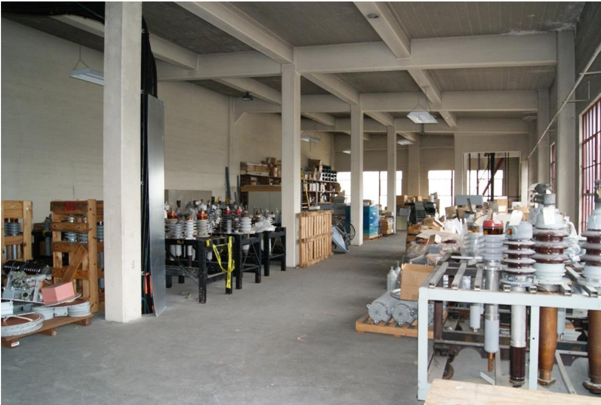
Photo 12 of 15. WA_PierceCounty_CushmanSubstation_0012. Second floor room at Cushman Substation, now used for storage.
