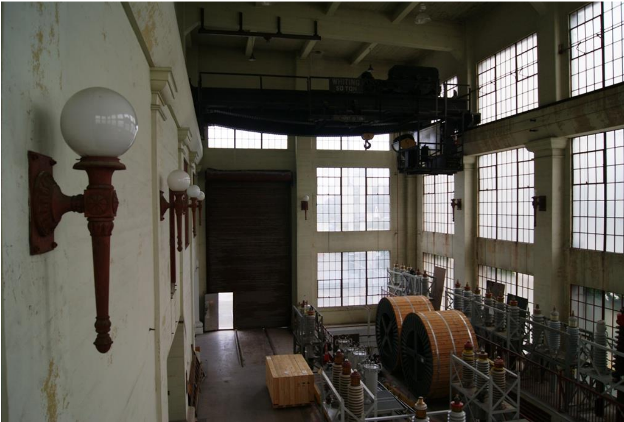
Photo 9 of 15. WA_PierceCounty_CushmanSubstation_0009. Interior of Cushman Substation, which is now used for storage. Note the decorative lighting, gantry crane (at ceiling), and voluminous interior space three stories high. Engaged pilasters are visible on both the south wall (pictured right) and interior wall (pictured left).
