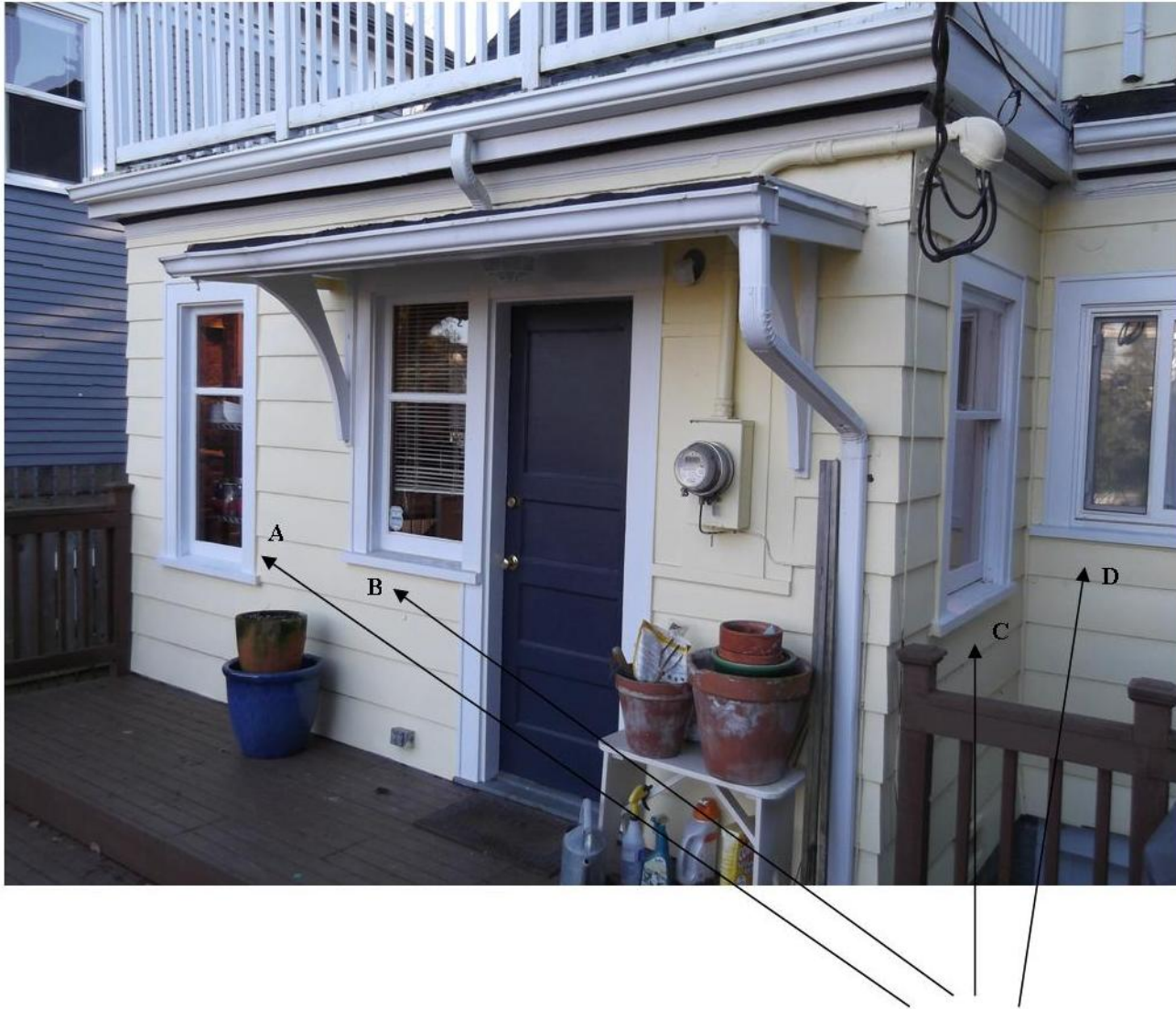
This picture illustrates more clearly the varying heights of window lines on existing “addition” structure that was not part of original structure. Noted: A,B,C windows to be replaced. Matching window height of window, D.
