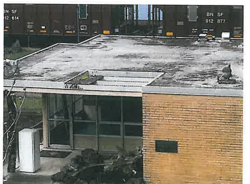
CITY OF TACOMA WESTERN SLOPES WASTEWATER TREATMENT PLANT #2: OPERATIONS BUILDING ROOF REPLACEMENT II ES15 - 0349N
