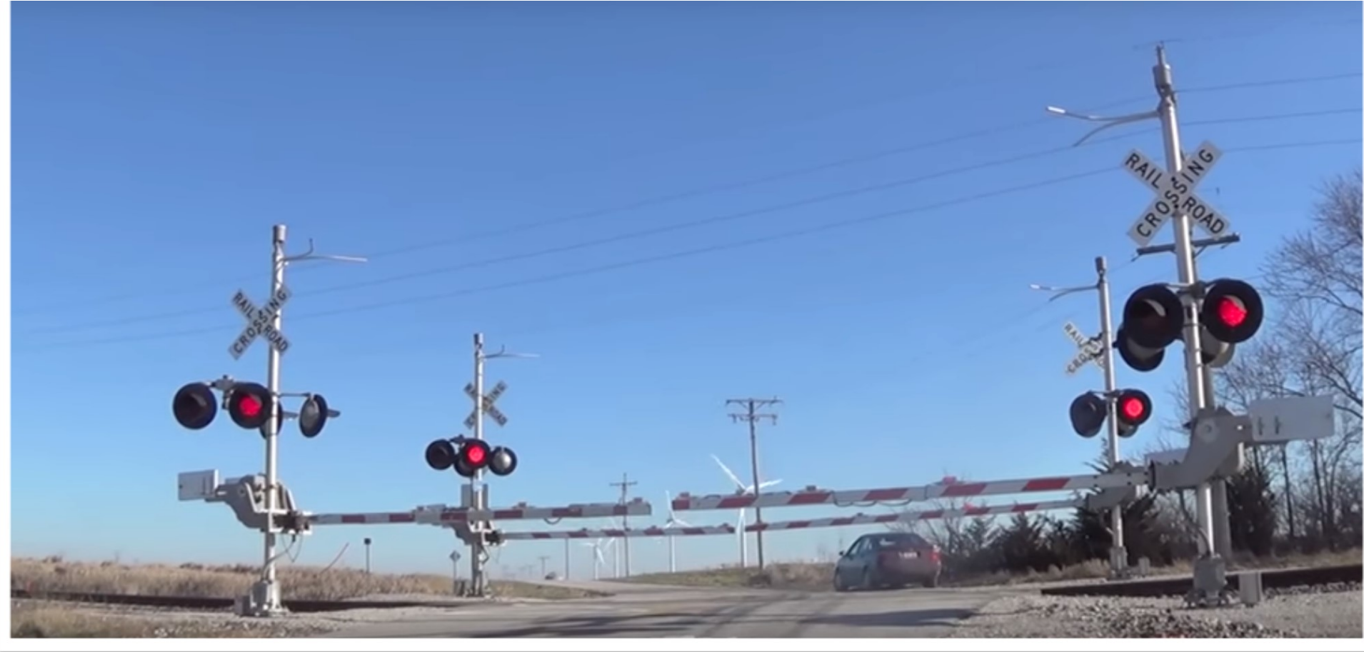
Example of a 4 quad gate system.
