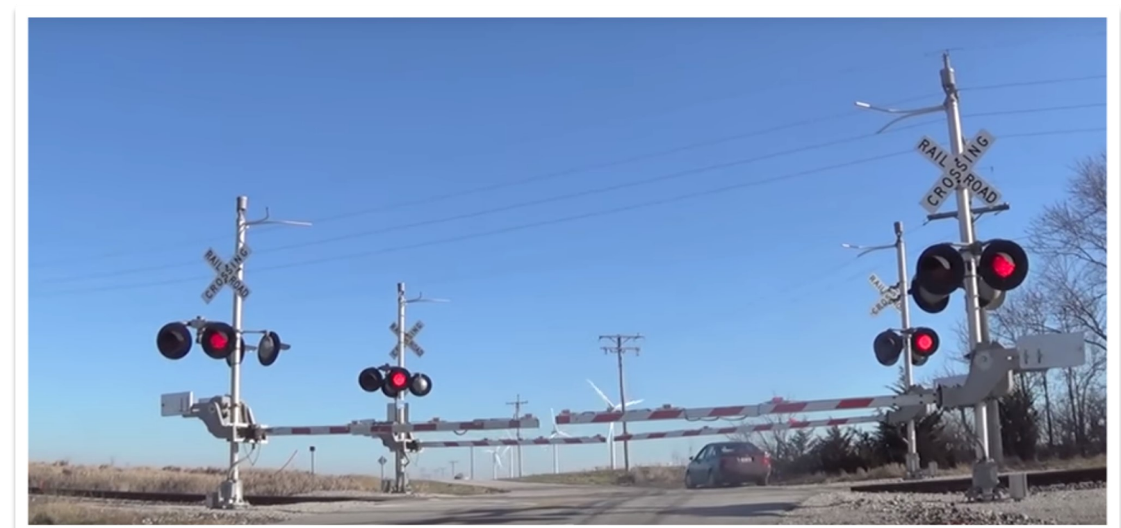
Example of 4 quadrant gates.
