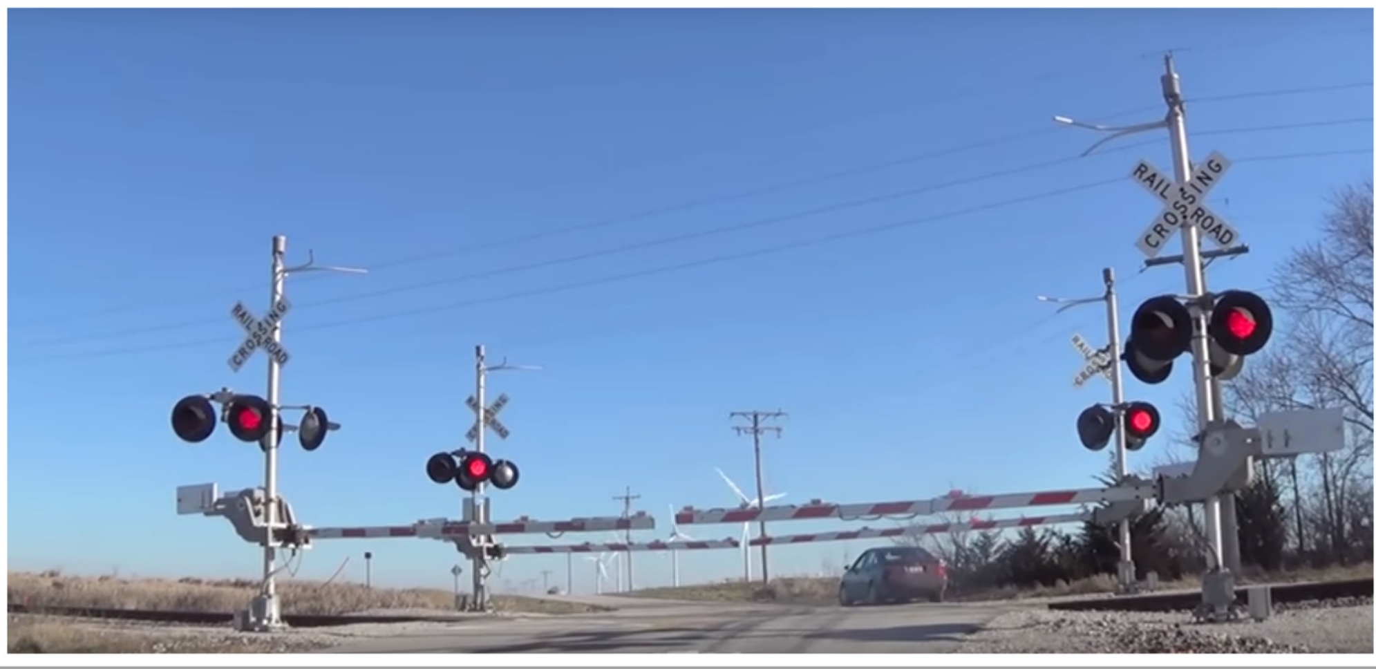
Example of 4 quadrant gates.
