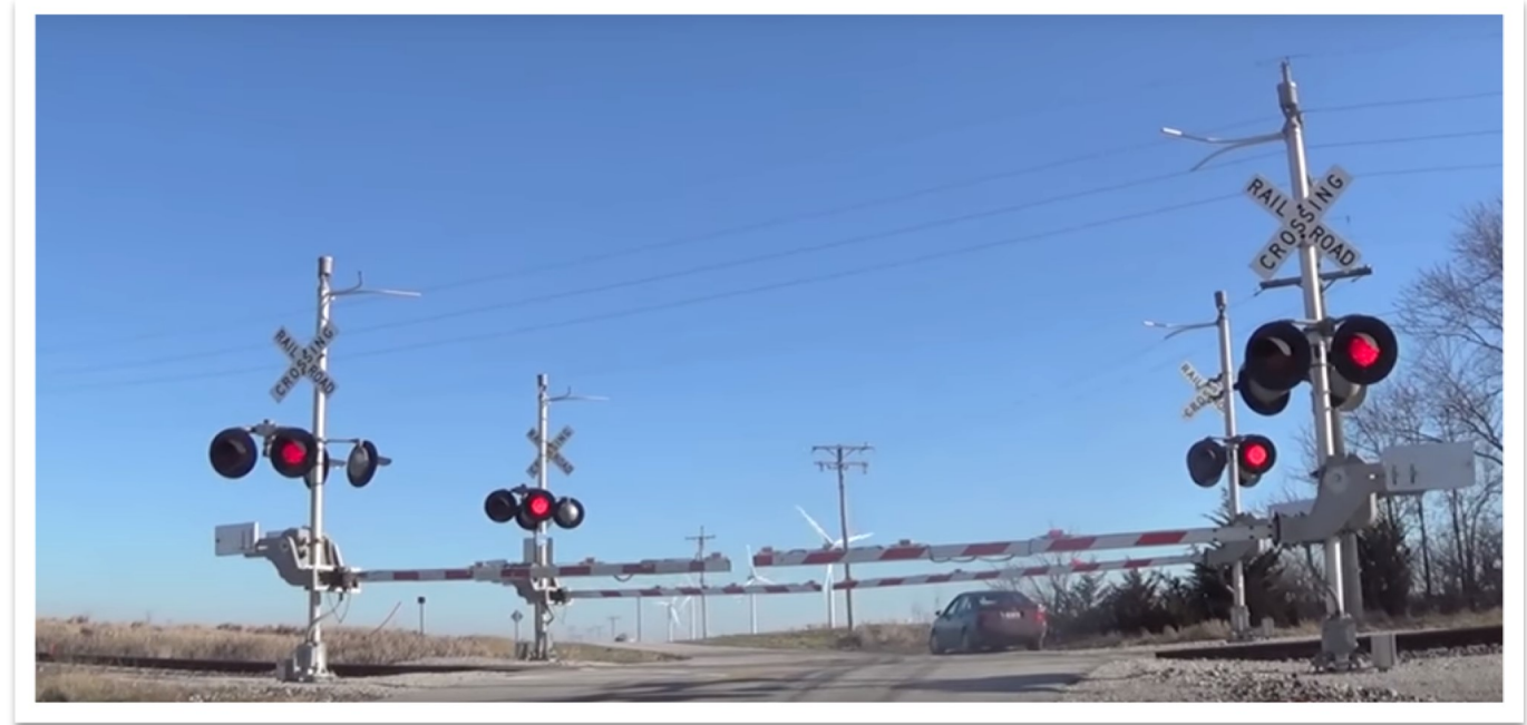
Example of 4 quadrant gates.
