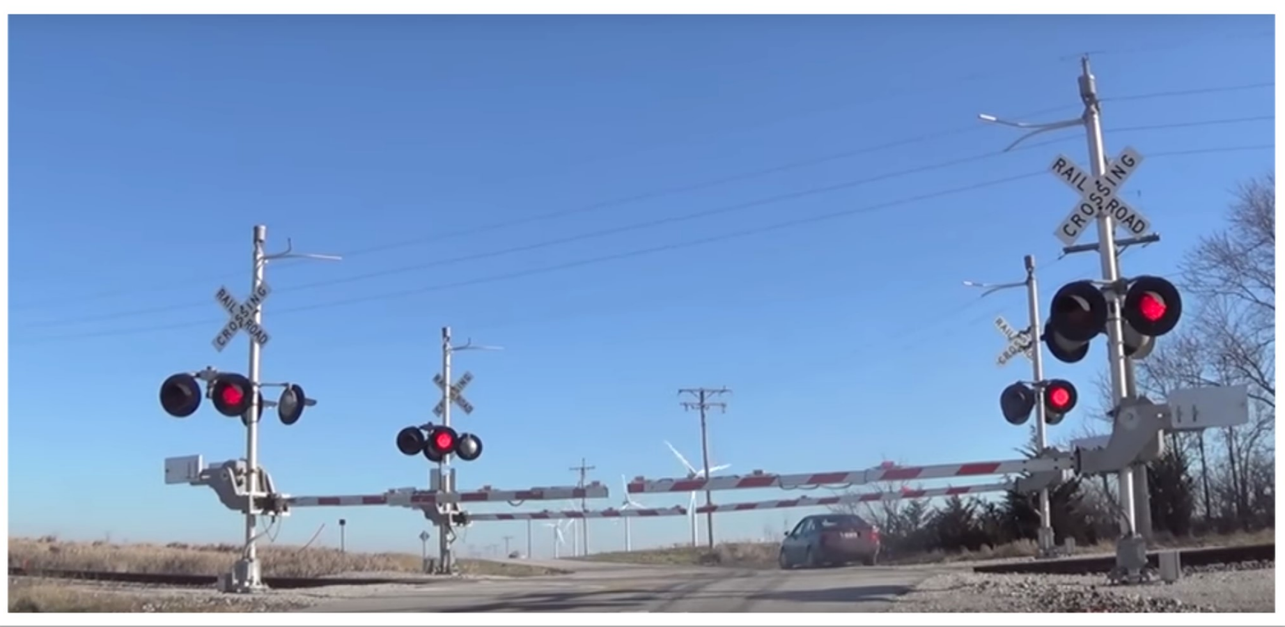
Example of a 4 quad gate system.
