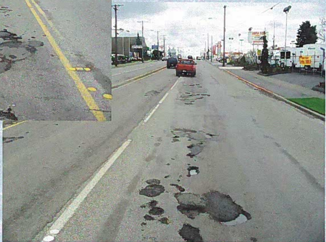
Roadway Surface Failures
