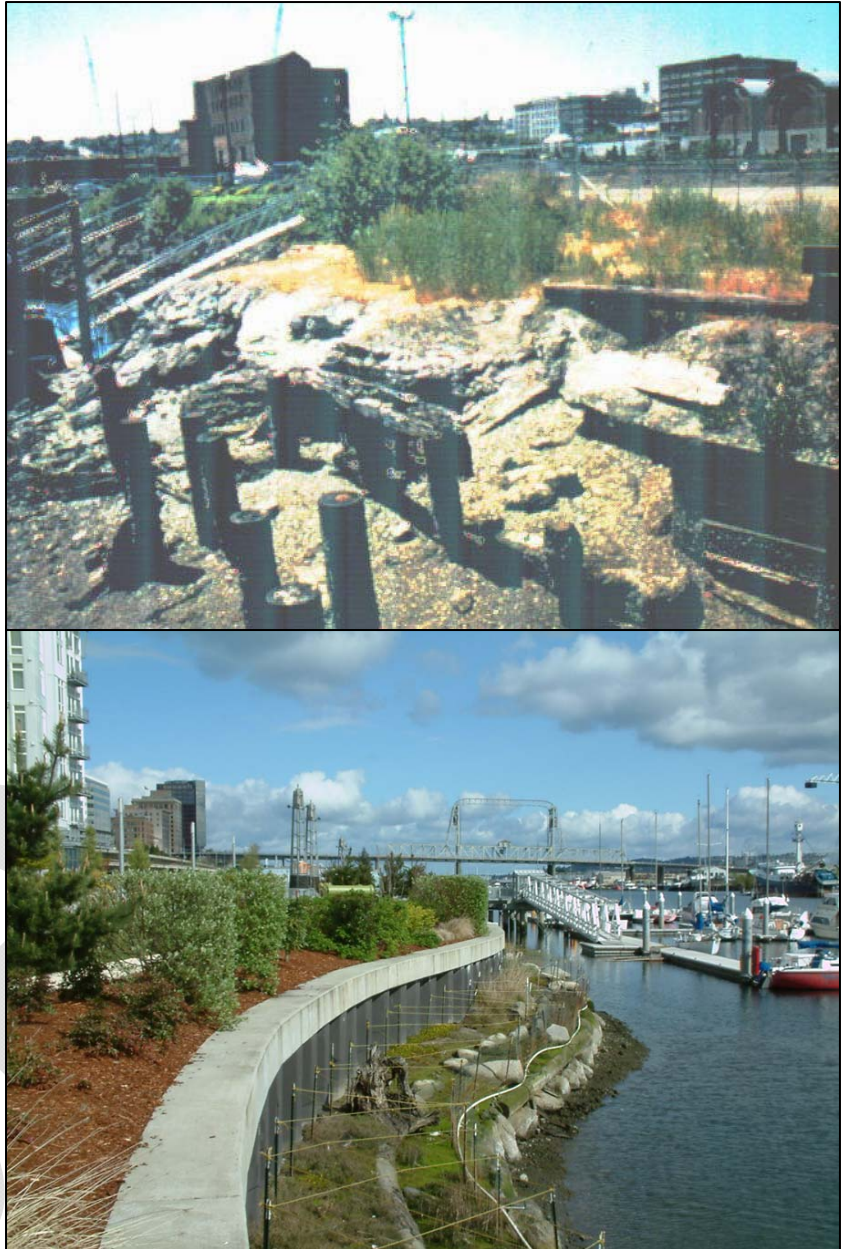
Figure 9 The top image shows a portion of the Thea Foss Waterway in 1998, before restoration activities. The bottom image shows the Thea Foss Waterway today. As shown, creosote pilings have been removed, a seawall was constructed to support the Thea Foss Esplanade and restoration plantings have been established between the wall and the water. This design provides an alternative to traditional shoreline armoring built directly at the shore. The shoreline vegetation between the bulkhead and water provide wave attenuation as well as overhanging native vegetation.
