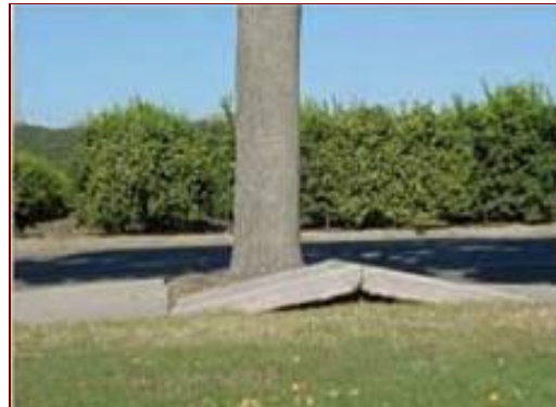
Subsurface tree roots can lift concrete sidewalk slabs, causing the surface to become uneven
