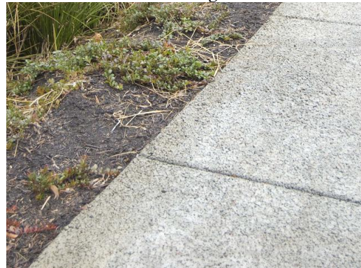
Permeable pavement can be used where drainage is an issue or where tree/sidewalk issues exist
