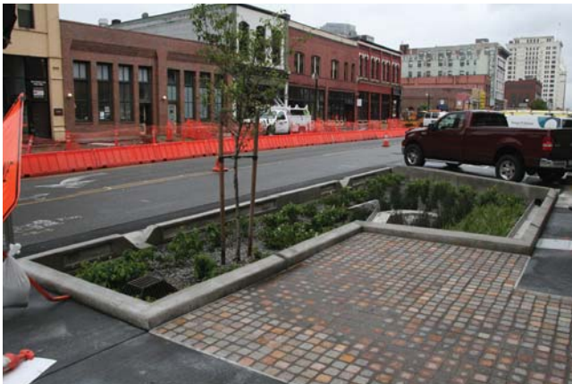
FIG. 8-11 The Pacific Avenue Streetscape project under construction. The project included the addition of fourteen rain gardens to pretreat stormwater before it enters the Thea Foss Waterway.
