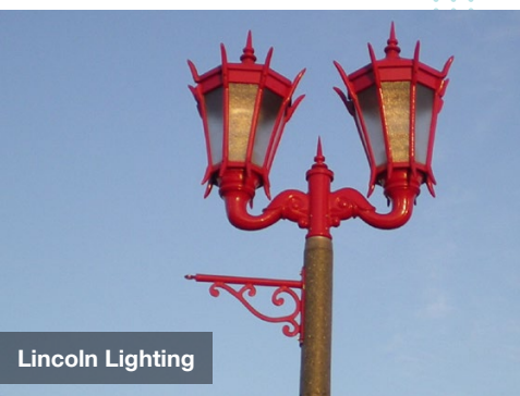
D Street Overpass Lighting
